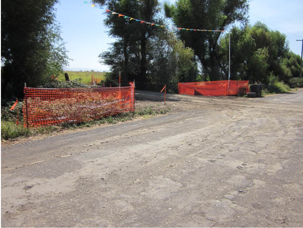
Photo 5: ESA fencing installed along northern side of D-6 (south side of Dodge Road) to protect sensitive habitat (Fremont Cottonwood Riparian Forest).
