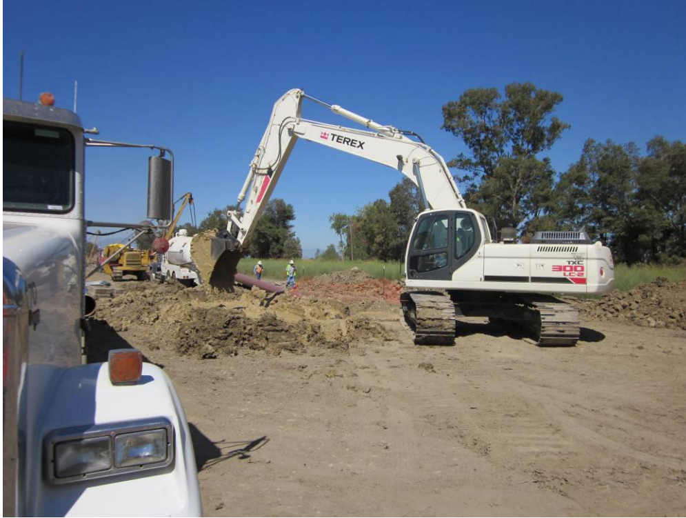
Photo 3: HDD at NRCS wetland. Drill mud being loaded into trucks for hauling offsite and treatment.
