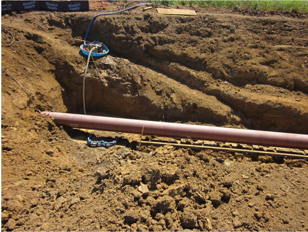
Photo 1: Auger bore at D-31. Pump containment in place and wildlife ramps installed.
