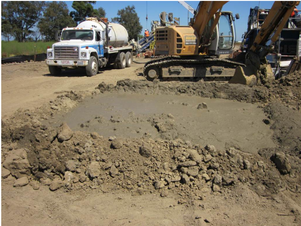
Photo 6: HDD at NRCS wetland. Frac-out material in foreground was contained under direction of the environmental monitor and hauled off-site for proper disposal.
